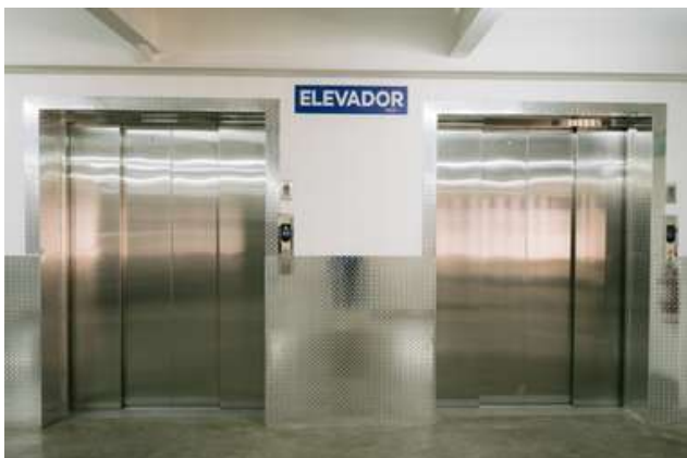
Load elevator and facility elevators
