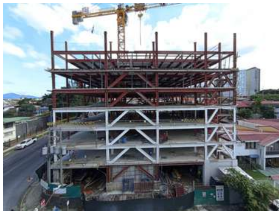
The steel structure under construction. In white, one can see the paint installed on the lower levels.
