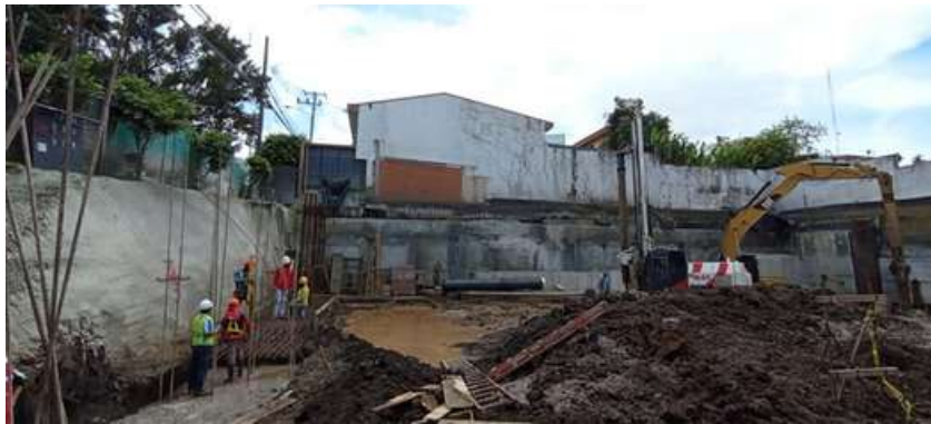
Retaining walls of the project. To the left, the soil nailing screen. Below the neighbor, the anchored wall.
